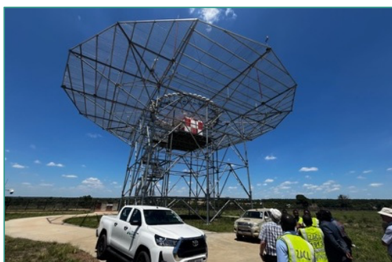
Instrument Landing System
